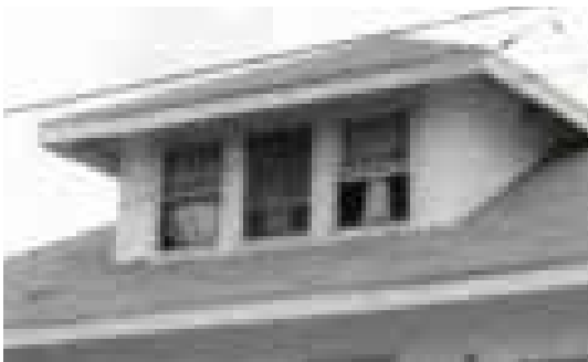
Windows in the dormer appear to have 6-lites on the top sash and a single light on the lower sash.
